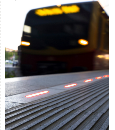
Illuminated platform edge on Platform 1 Berlin Südkreuz Photo: DB / H.-C. Plambeck
